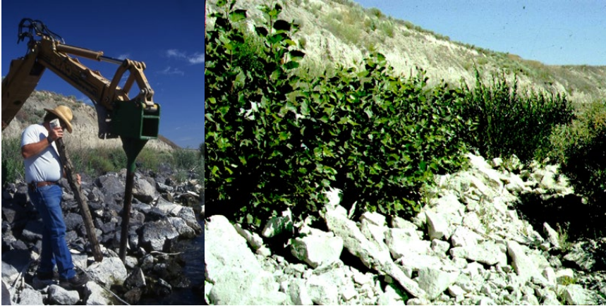
Figure 16-10: Live Pole being installed through riprap with a stinger (left) and after 3 years.
